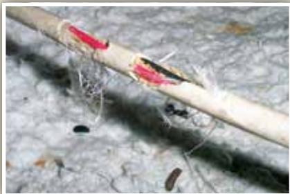
Gnawing on wires with droppings.*
