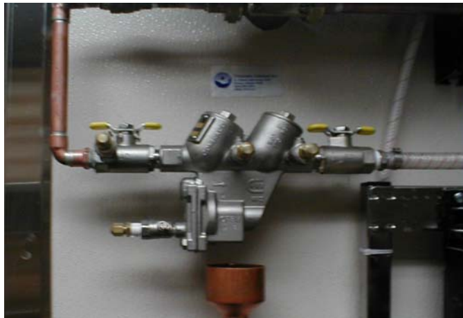
Figure 8. RPZ on Carbonator Supply Line
