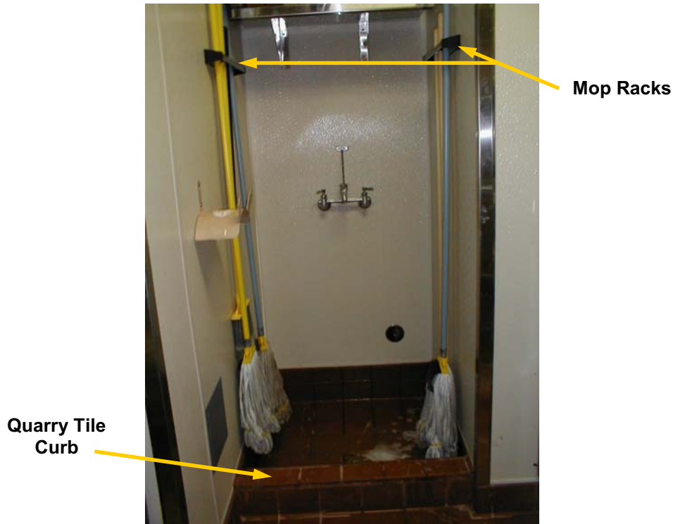
Figure 6. Quarry Tile Mop Sink / Janitorial Station
