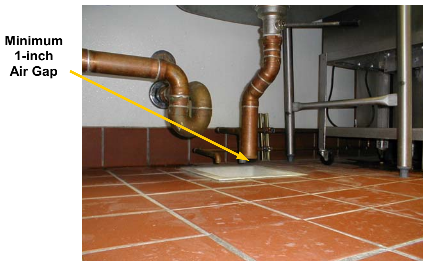
Figure 9. Air Gap On Food Prep Sink
