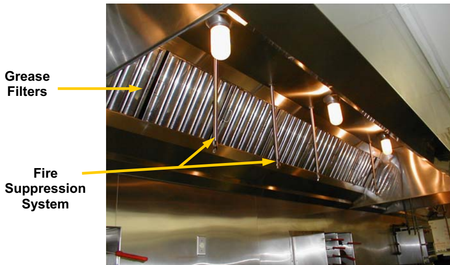
Figure 12. Type I Hood Over Cook Line
